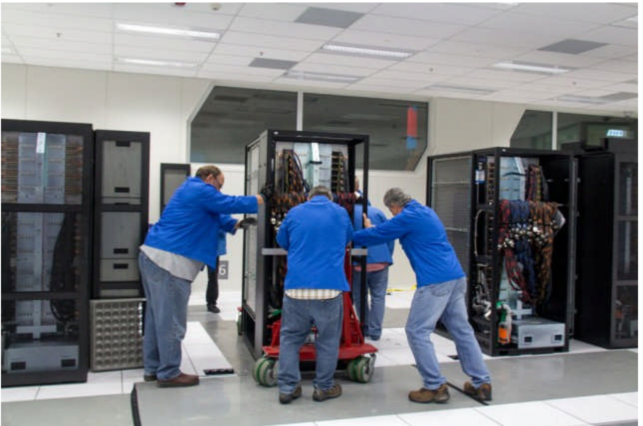
Wheeling the XC30 supercomputer into place
